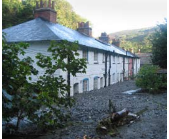
The impact of flooding in Boscastle, Cornwall. Climate change is having a detrimental effect on our way of life
